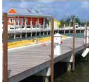
Phase I :: Close to completion and includes core facilities like the marine docks, fuel station and Changing rooms
