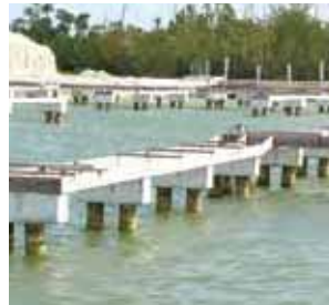
Phase I :: Marina docks, fixed concrete and hardwood with power and water at every slip
